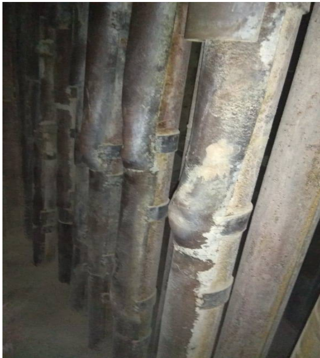
Figure 1 Bulging found in rear arch sleeves and tubes
