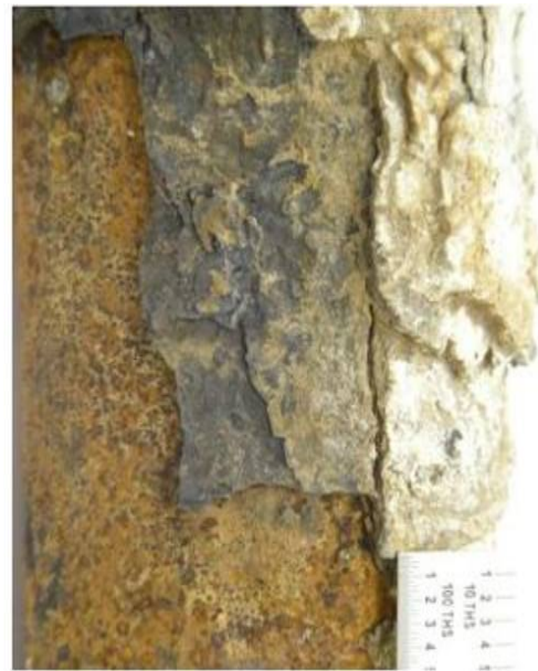
Fig-7. Photograph of super-heater tube surface with thick deposits due to corrosion (5)
