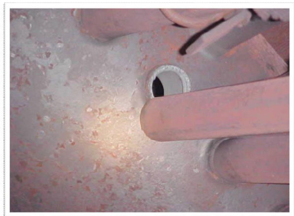
Damage to attachment cleats
