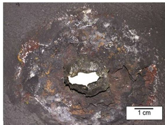
Fig-9. Caustic corrosion failure of tube. It shows white color deposits near the rupture (9)
