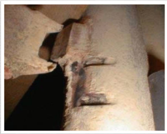
Damage to header stub
