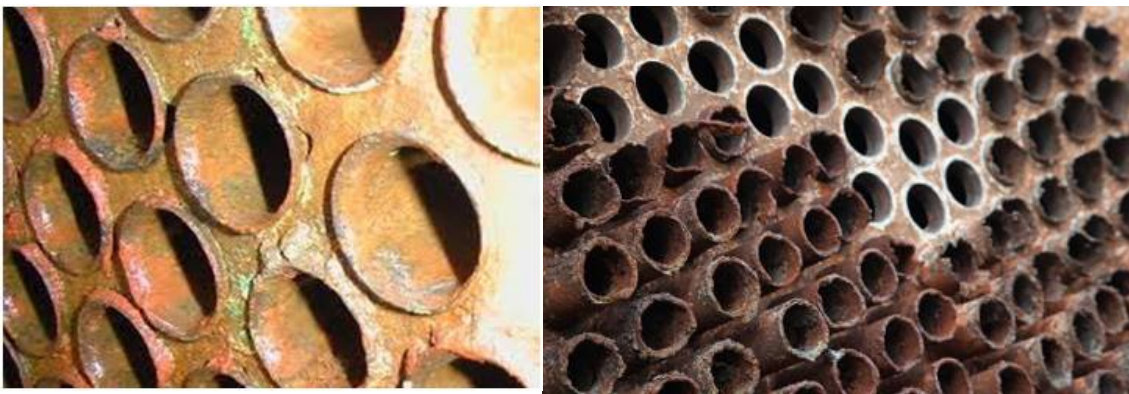
Fig. Boiler Tube Galvanic Corrosion
