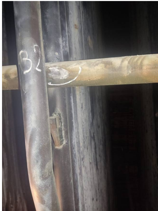
Figure 3 Mechanical rubbing observed in PSH tubes with spacer tubes
