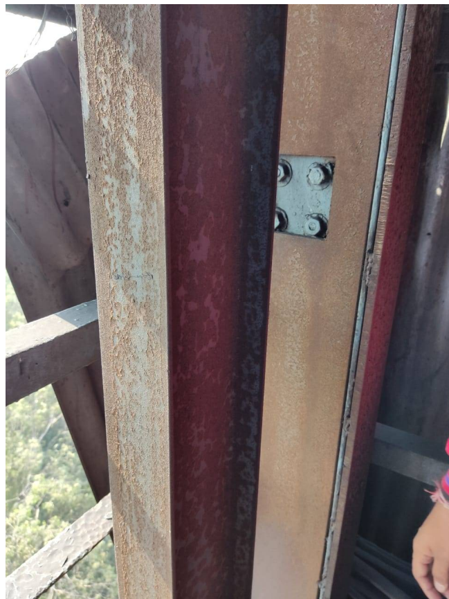
Figure 2 Corrosion in secondary coal crusher
