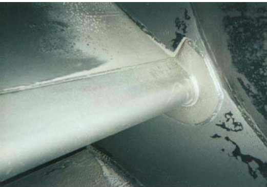
Fan Liner protected with WRTPL's XL-800FC in the same application after 12 months service.
